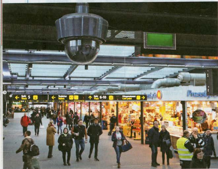
An Axis network camera system in use at Malmö Central Station in Sweden
