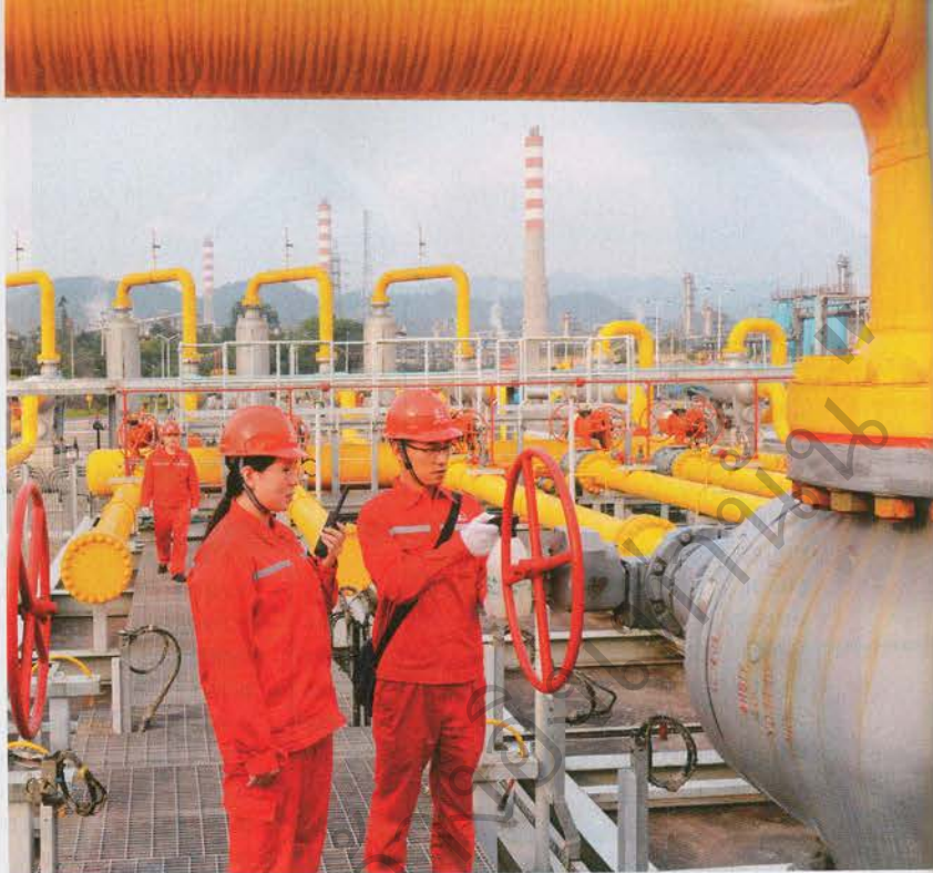
Sinopec workers at a natural-gas purification plant in China's Sichuan province.
